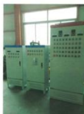
电控箱 Electricity Control Cabinet
